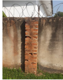
Wall - needs paint Post - needs cement
