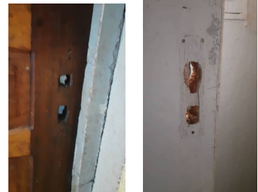
Missing Door Locks
